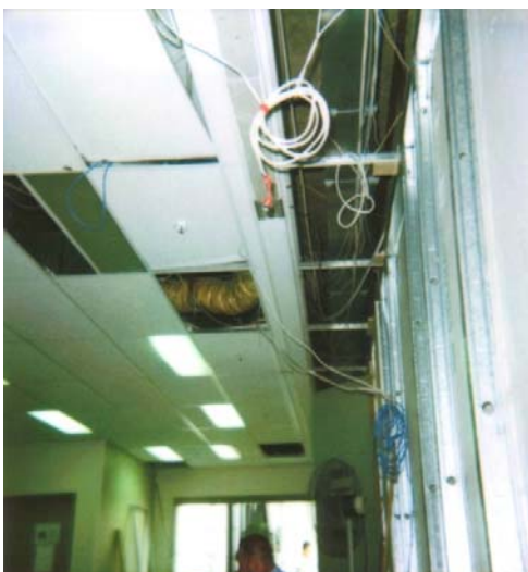
Fig 5. Some of the 22 missing ceiling tiles.
