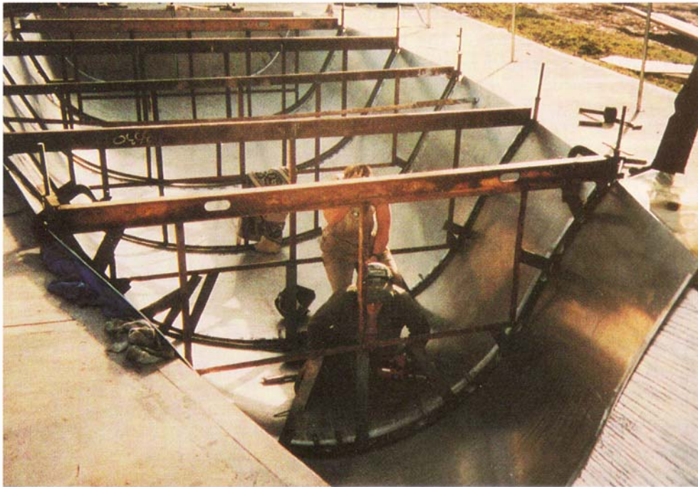
A steel frame was used to hold the aluminium sheets in position in the mould during welding
