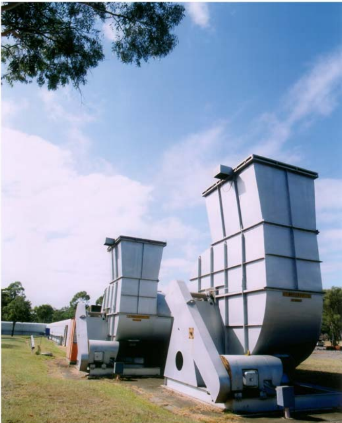
Gallery exhaust fans which controls the rate of air flow
