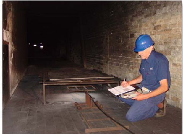
Laurie Gerisch checking the temperature & humidity of the air flow through the gallery
