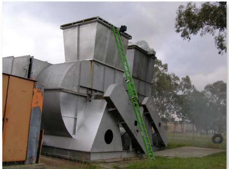
Refurbished fire gallery fan assembly
