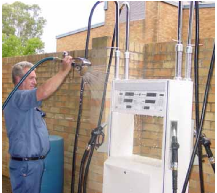
Senior Electrical Technical Officer Les Golder conducting an IP test on a fuel dispenser
