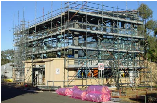
Building 13 roof and cladding stripped
