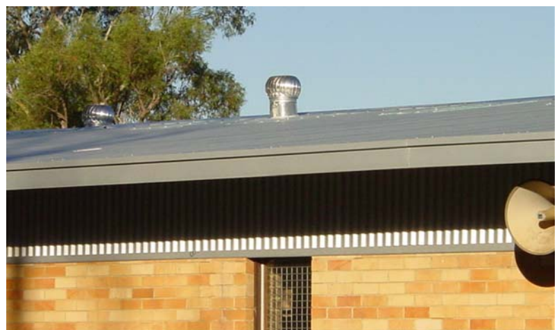
Building 10 showing new roof and vent with side AC louvre vents replaced with fixed cladding
