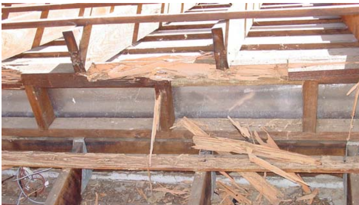
Building 8 old termite damage revealed by the storm
