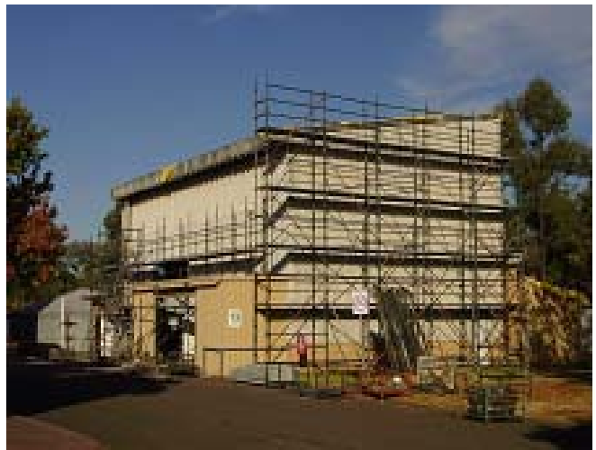
TestSafe's Mechanical Testing Building becomes Asbestos free (note the worlds biggest asbestos eaves gutter)
