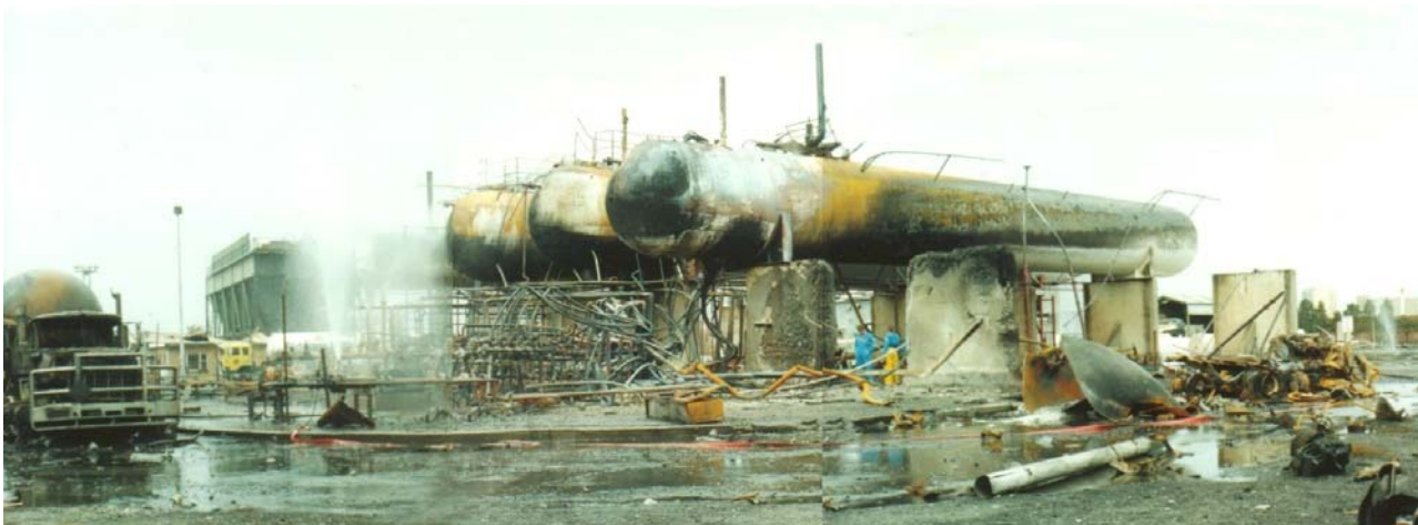
View of the LPG terminal after the explosion. Note: damaged manifold and pipes (centre left), Tank No 1 missing (centre right), remains of the destroyed LPG Road Tanker (far right) and discharge pipes from the PRVs on the top of each tank
